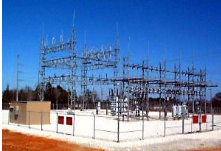
Figure 4.8 Distribution substation [OSHA, 2016]
